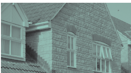
Type G cavitytrays with attached lead flashings provide protection to the front horizontal intersection. Note the Type X trays used above the sloping abutment terminate with an external angle. This provides a protective link with the Type G trays.
